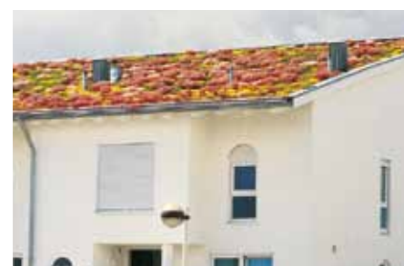
A shear barrier is placed just above the eaves on this monopitch roof, which is drained by means of an outer-lying gutter.
