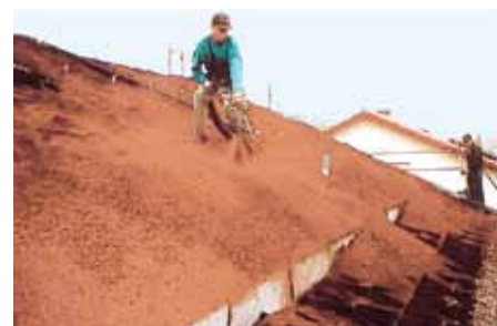
The system substrate “Heather with Lavender-light” is, e.g. delivered in a silo tanker. It is then blown onto the roof using a hose until the Georaster® elements are filled and covered up to about 10 mm over their upper edge.
